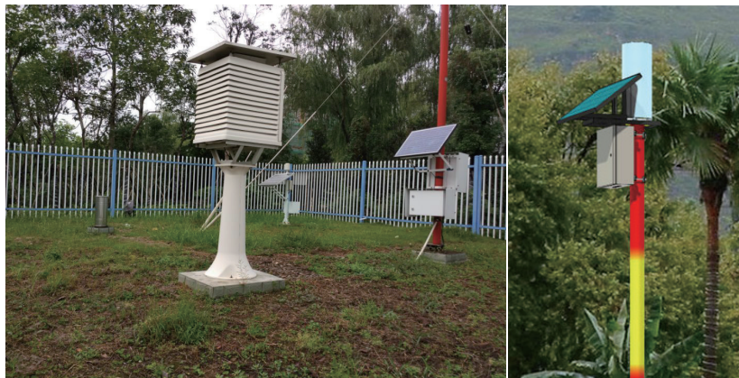
Fig. 2. (Color online) Automatic rainfall monitoring station.
