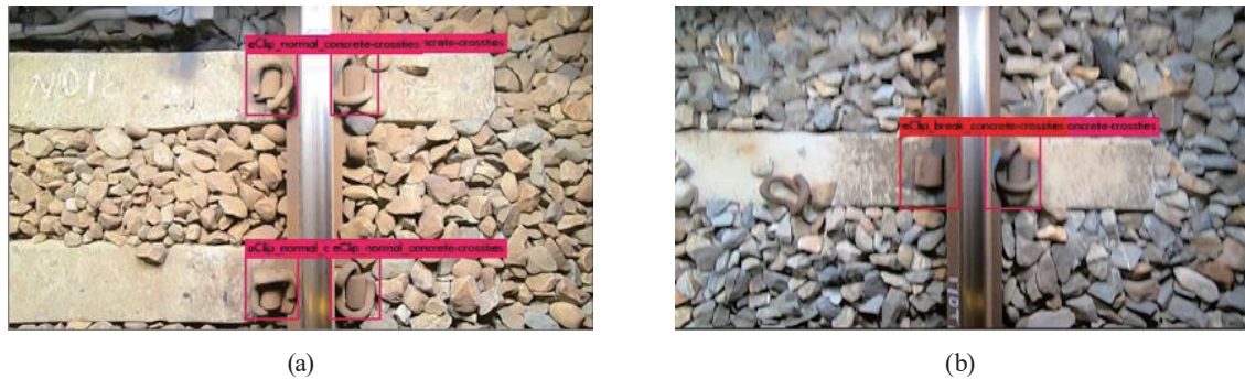
Fig. 6. (Color online) Some test images. (a) Normal e_clips on concrete cross-tie. (b) Left e_clip is missing while the e_clip on the right is normal.
