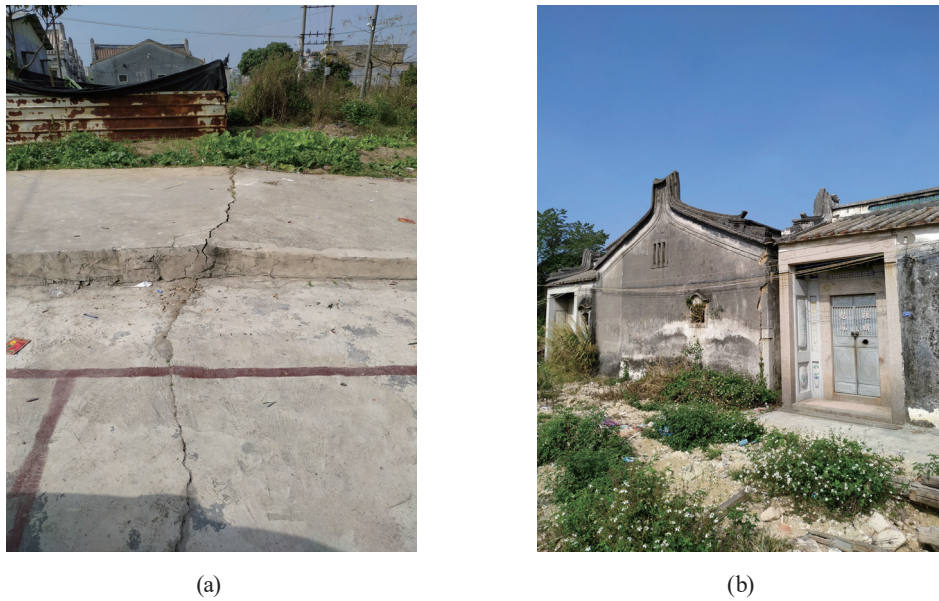
Fig. 5. (Color) Ground fissures and house crack in ground uplift area edge. (a) Ground fissure and (b) crack in house.
