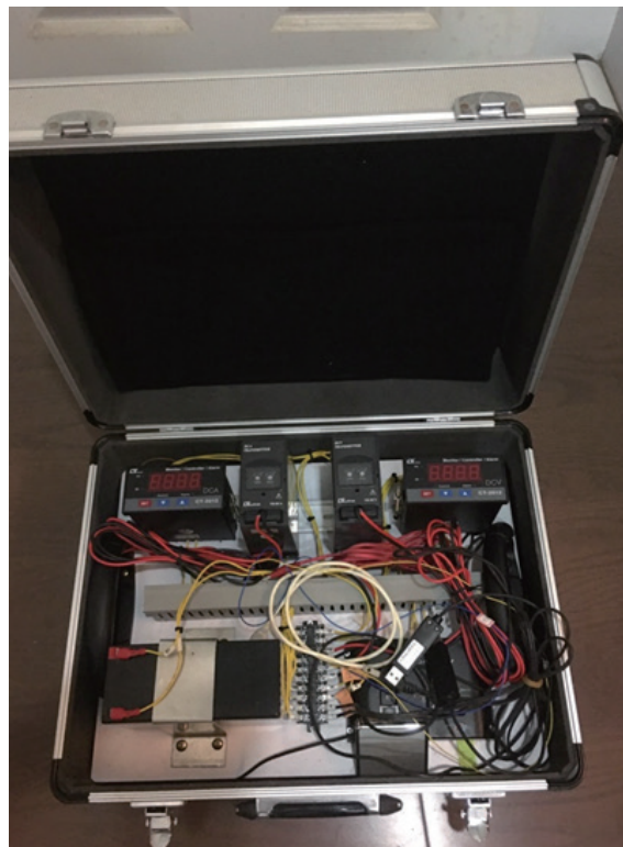
Fig. 11. (Color online) Control unit of using and charging battery.
