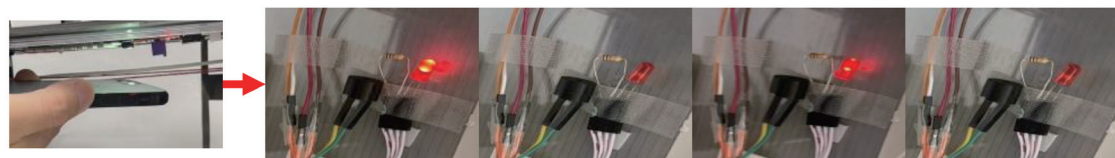
Fig. 8. (Color online) Testing of the alarm and warning light functionality.
