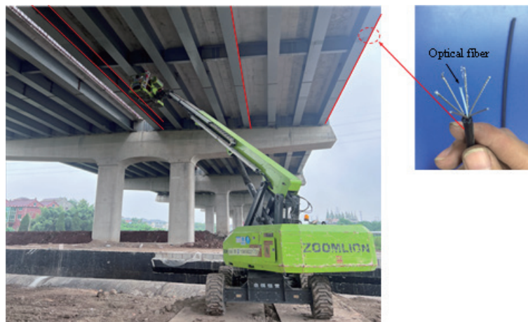
Fig. 8. (Color online) On-site photograph of the distributed optical sensing fiber installation.
