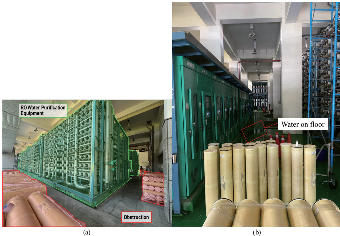
Fig. 14. (Color online) Test environment: (a) dense RO equipment and (b) leaked water on floor.
